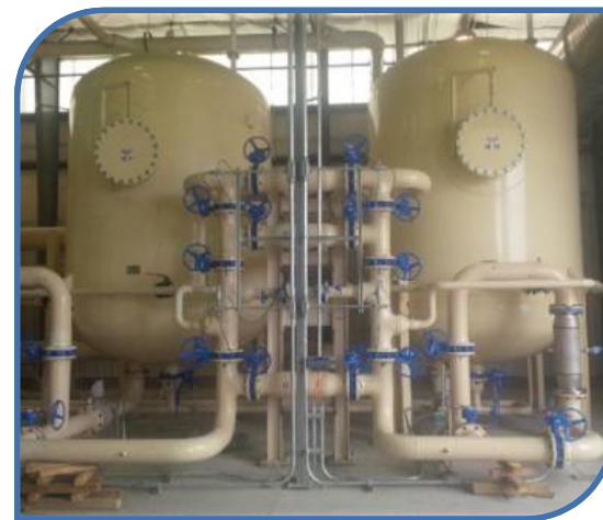
Ion Exchange Vessels for Uranium Recovery
