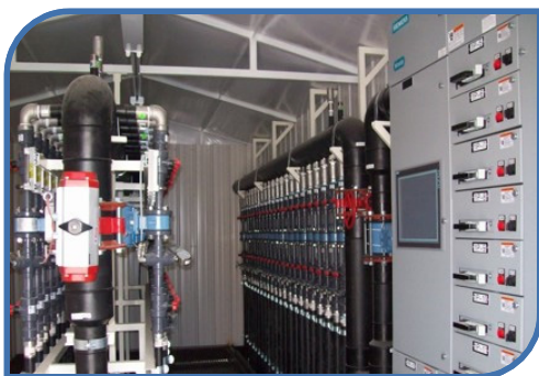
Interior of Header House
